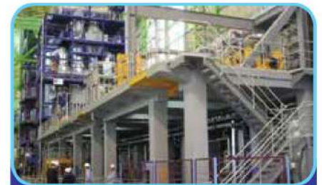
Strip Zinc Coating Line
